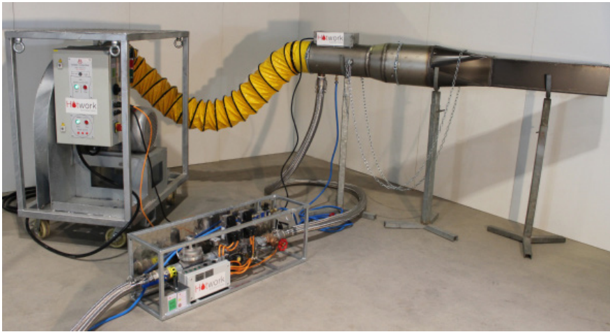
HV3000 with Silencer and Filter installed on a Float Furnace Doghouse
